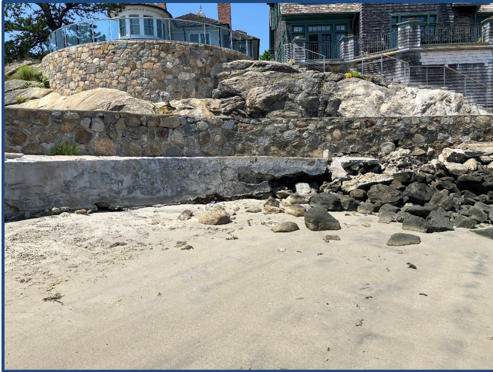
Figure 7: Severely Deteriorated Lower Seawall Adjacent to Stone Revetment, Facing North (6/17/2025)
