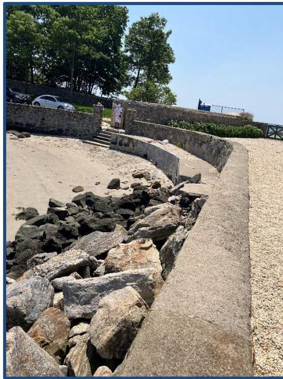
Figure 6: Former Deteriorated Lower Seawall, Facing Southwest (6/17/2024)
