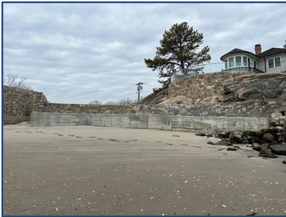
Figure 2: Repaired Lower Seawall as Seen from Waterward Edge of Beach, Facing West (3/4/2025)
