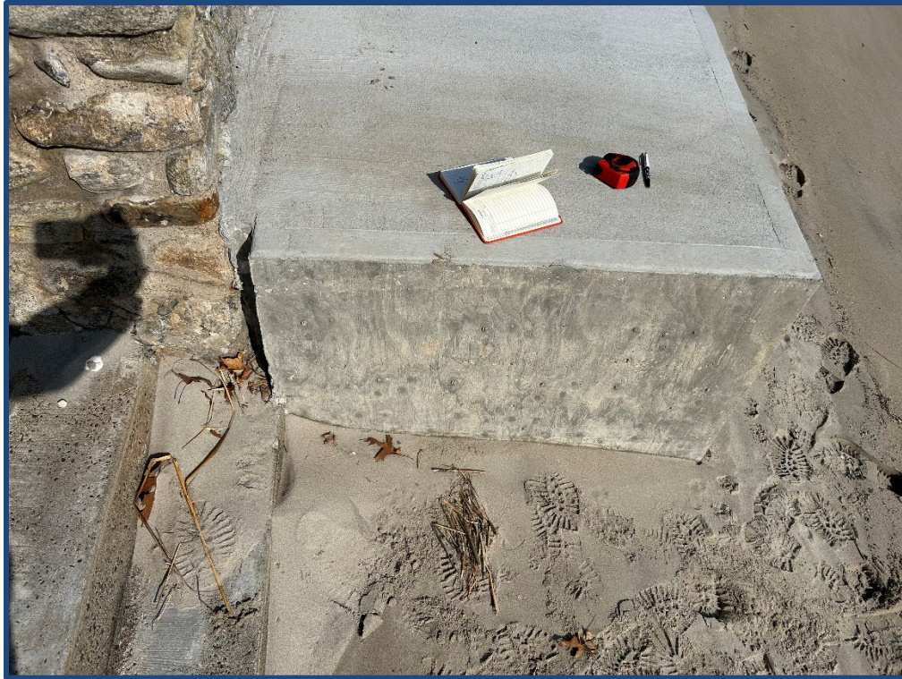
Figure 5: End Of Lower Seawall Adjacent to Stairs, Facing Northeast (3/4/2025)
