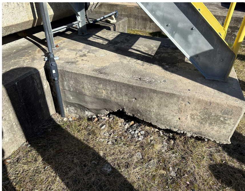
#16 -External Fuel Tank Stairs - Damage Close up
