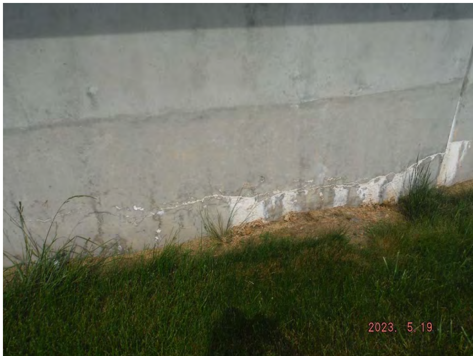
Tank #1 - Outside face of Segment #4-3, looking west. Note longitudinal hairline crack at lower wall.
