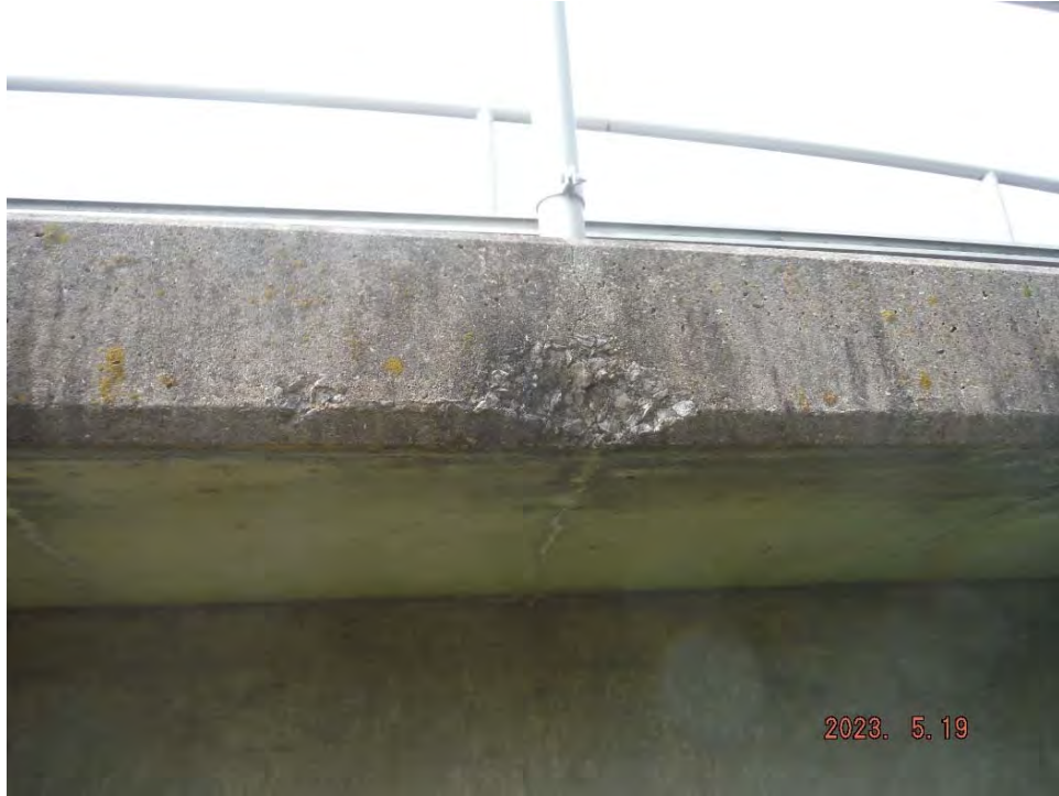
Tank #1 - Small (1/4 SF) shallow spall at fascia of catwalk at Segment 11-12, looking south.
