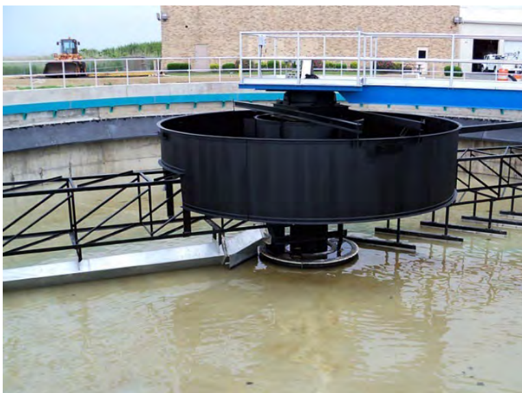
Figure 3. Suction Header Type Clarifier from Envirodyne Systems Inc.
