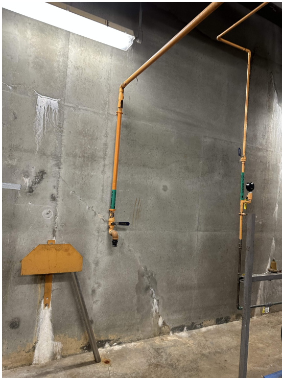
#3 -Efflorescence on Wall
