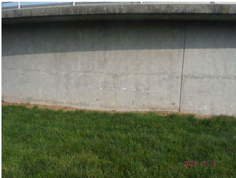
Tank #4 - Outside face of Segment 6-7, looking northeast. Note longitudinal hairline crack at the lower wall.
