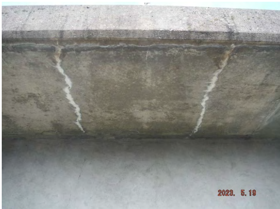
Tank #3 - Bottom of catwalk at Segment 5-4, looking northwest. Note transversal hairline cracks with efflorescence.
