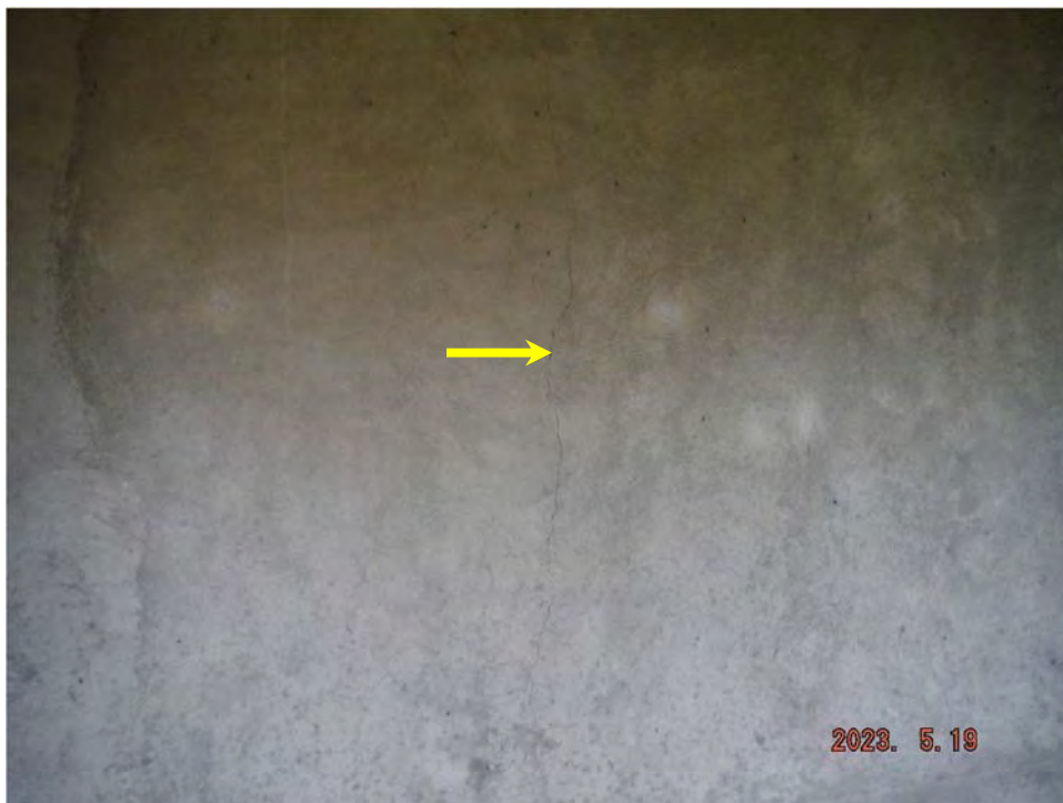
Tank #2 - Outside face of Segment 10-11, looking south. Note vertical hairline crack.
