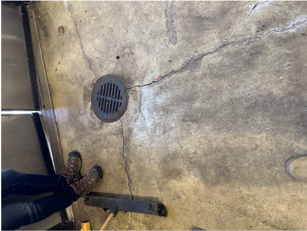
#13 -Cracked Topping on First Floor
