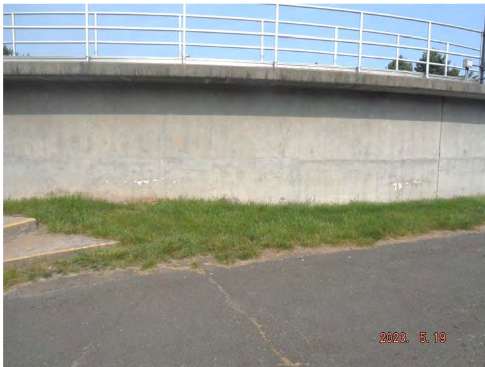
Tank #3 - Outside face of Segment 6-5, looking north. Note longitudinal hairline crack with efflorescence at lower wall.
