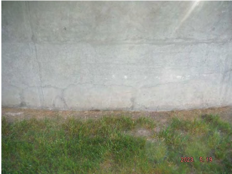
Tank #4 - Outside face of Segment 7-8, looking northeast. Note longitudinal hairline crack at the lower wall.
