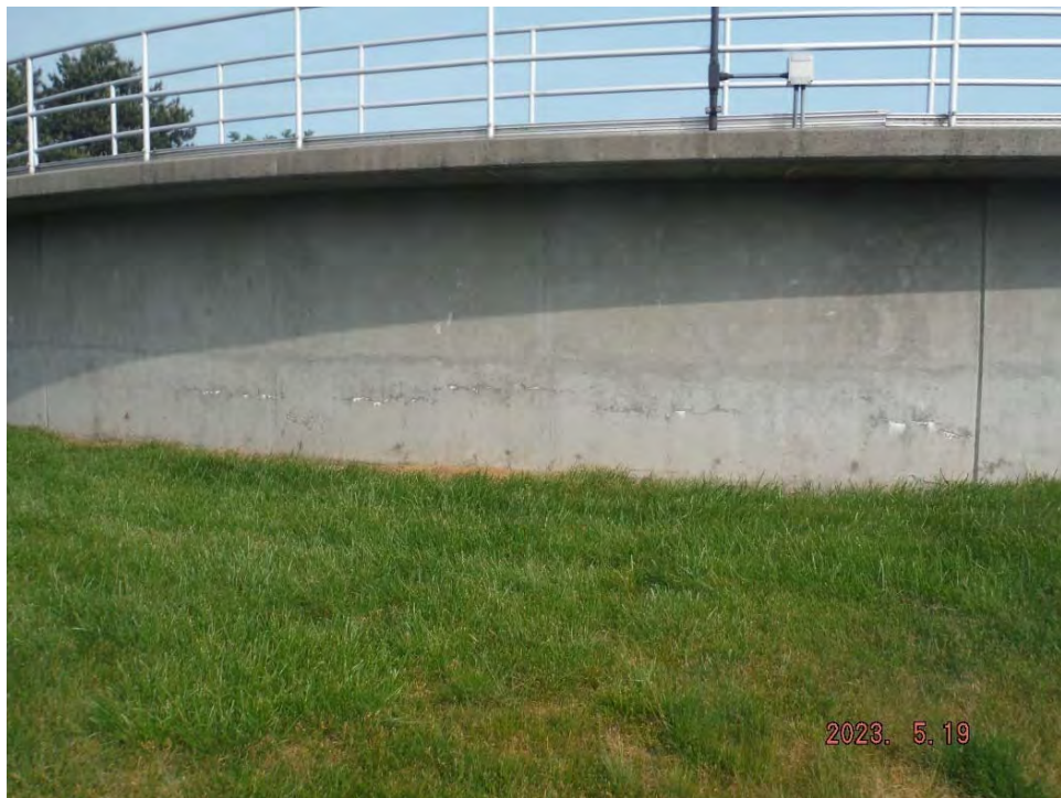
Tank #2 - Outside face at Segment 6-7, looking north. Note longitudinal hairline crack with efflorescence at lower wall.
