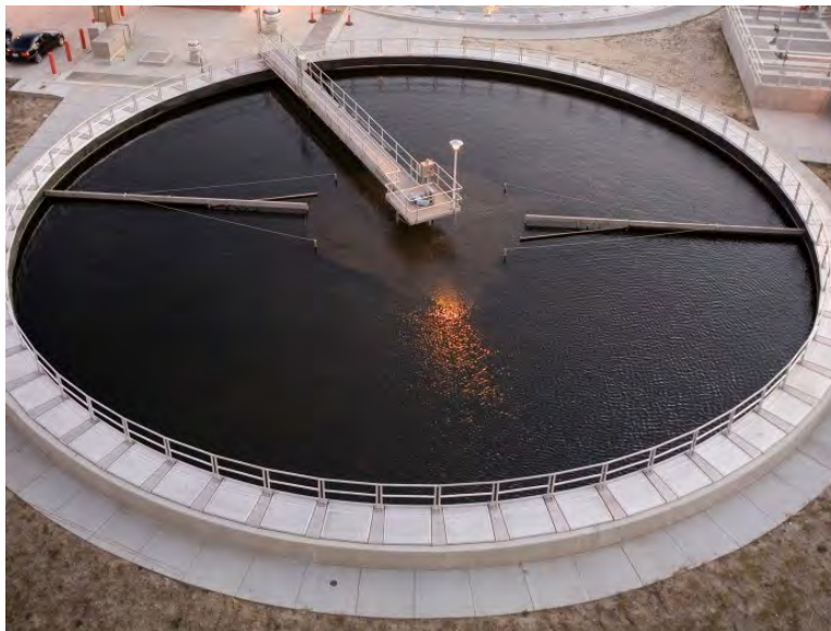
Figure 9. Hallsten Aluminum Effluent Launder Cover
