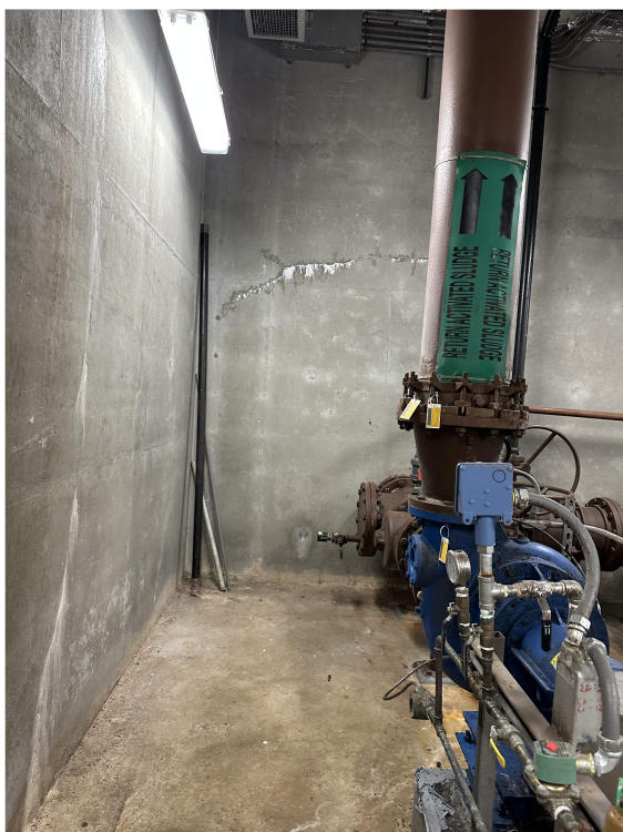
#7 -Efflorescence on Wall
