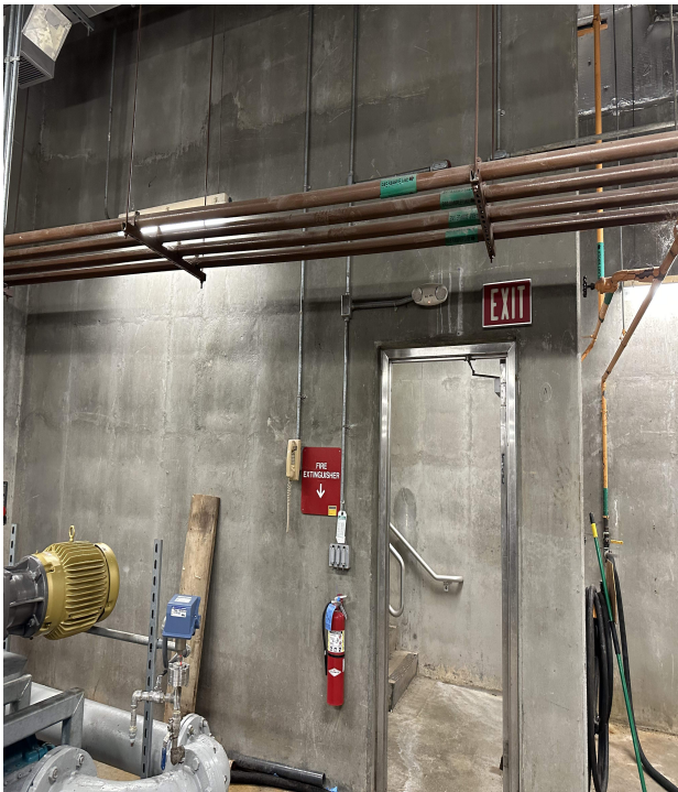
#9 -Efflorescence on Wall
