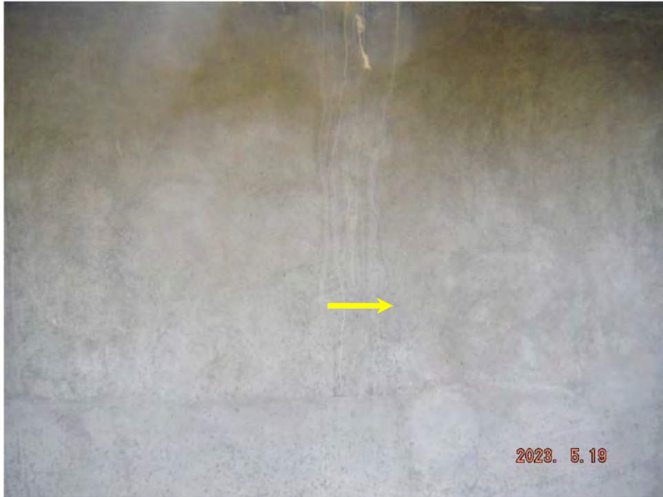
Tank #3 - Outside face of Segment 11-12, looking south. Note vertical hairline crack.
