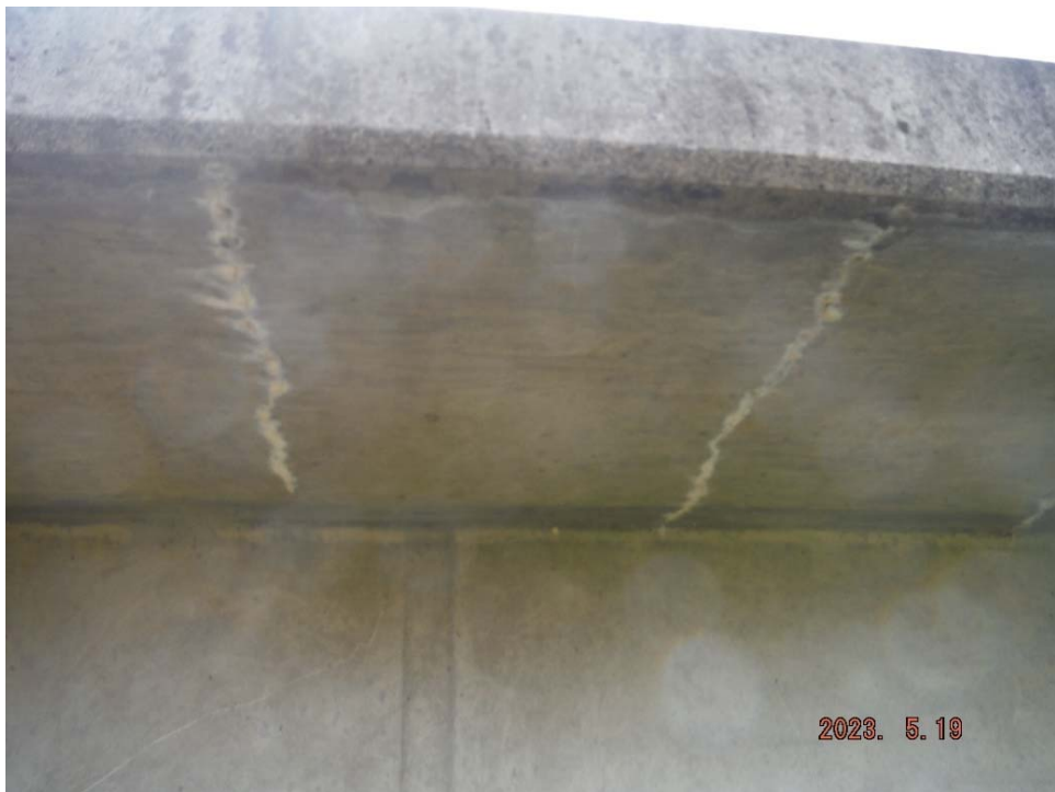
Tank #4 - Bottom of catwalk at Segment 12-1. Note transversal hairline cracks with efflorescence (typical for all segments, all tanks)
