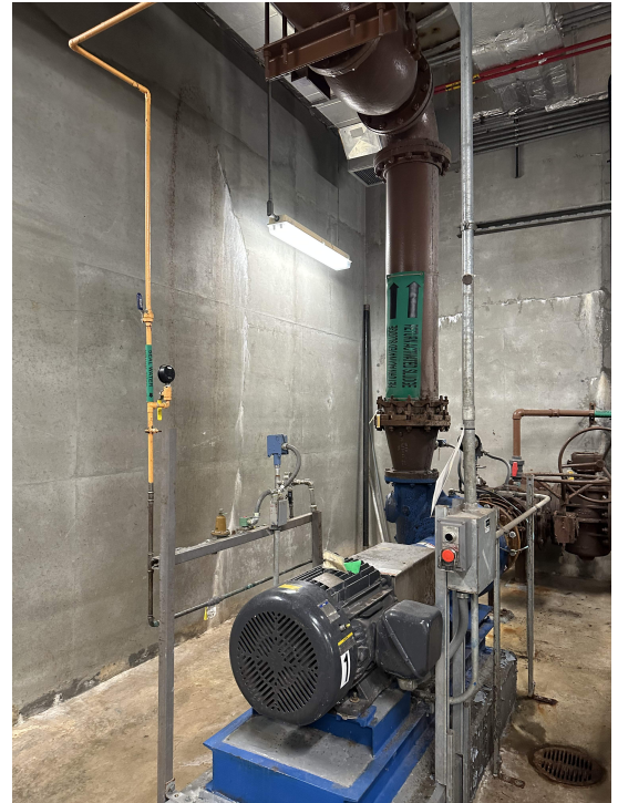
#4 -Efflorescence on Wall
