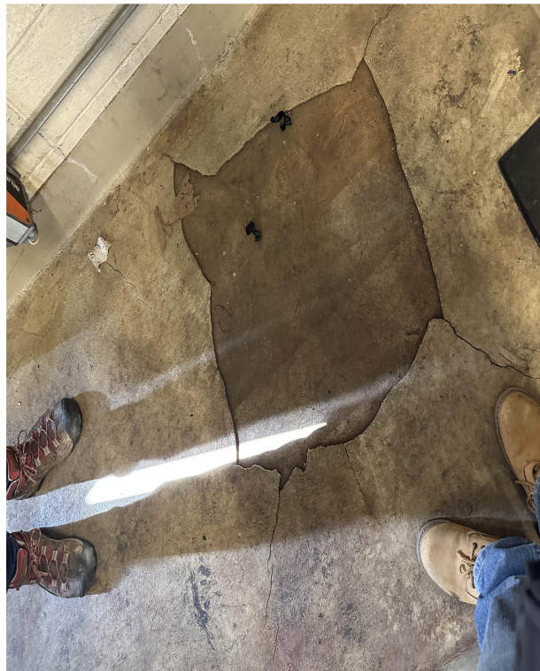
#14 -damaged Topping on First Floor
