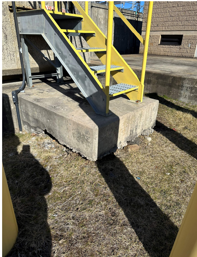
#15 -External Fuel Tank Stairs - Damage
