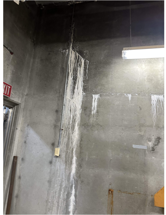
#2 -Efflorescence on Wall
