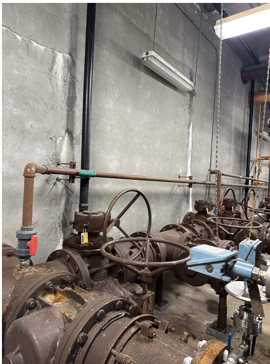
#5 -Efflorescence on Wall
