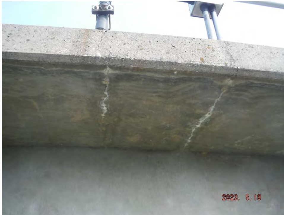
Tank #2 - Bottom of catwalk at Segment 6-7, looking north. Note transversal hairline cracks with efflorescence.
