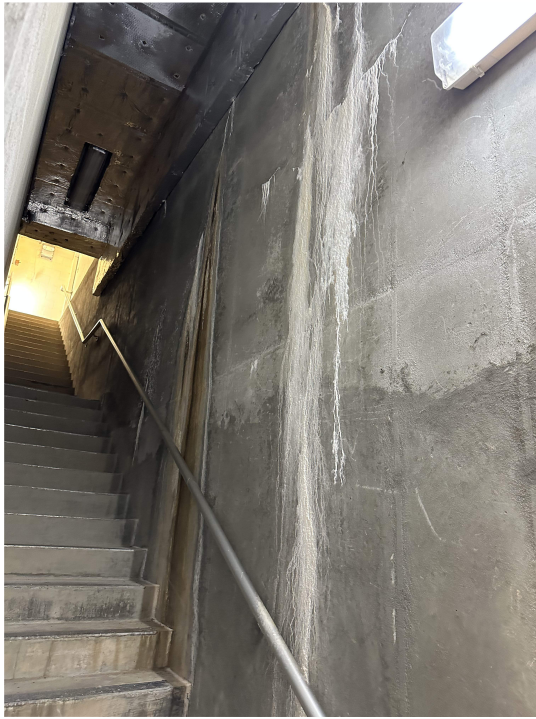
#1 -Efflorescence on Wall
