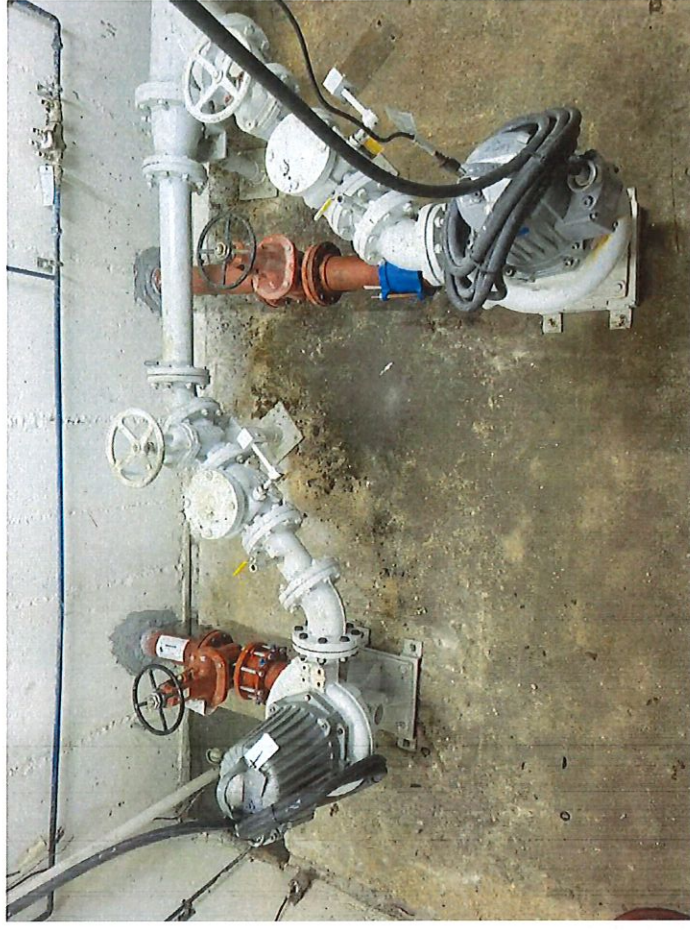
New 6" suction piping and valves
