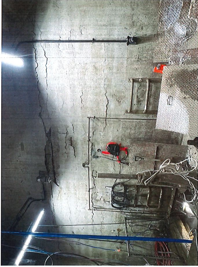
Concrete chipping on walls above wet well area - require concrete repair work
