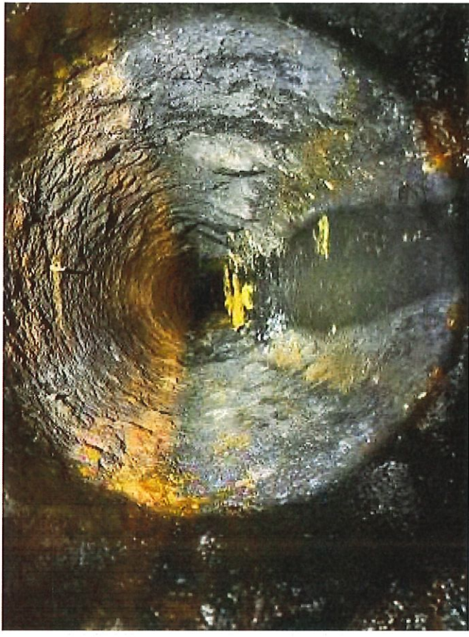
Existing gravity sanitary sewer pipe (3 segments) is in poor condition – requires CIPP Lining
