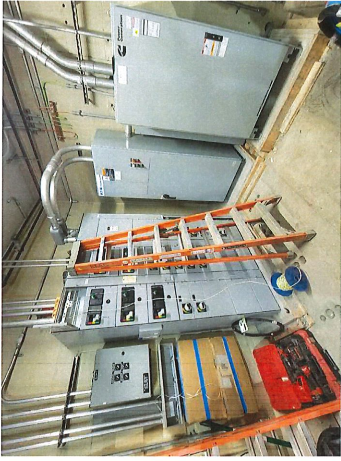
New electrical equipment including MCC, temperature control, and lighting control panels
