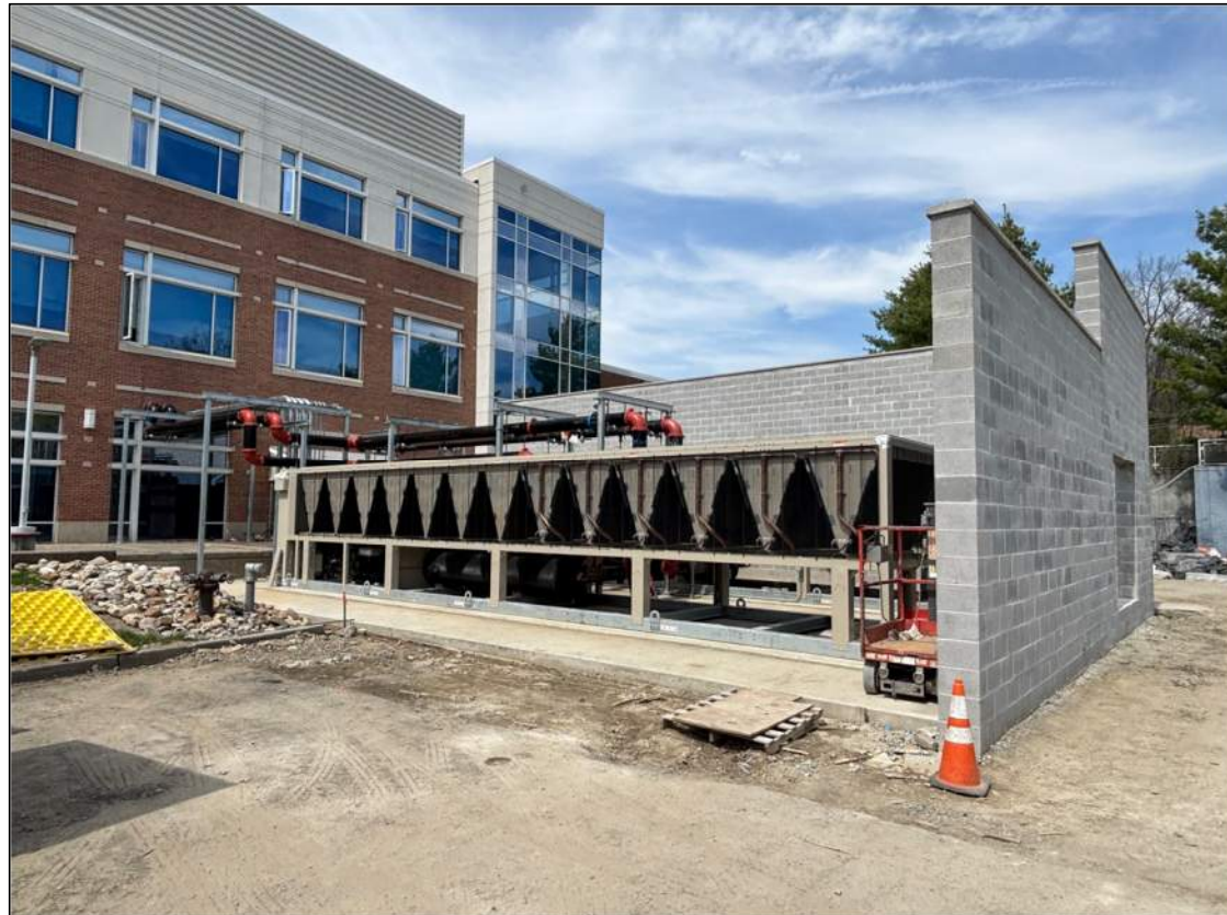
New Outdoor Chiller – 4/16/26
