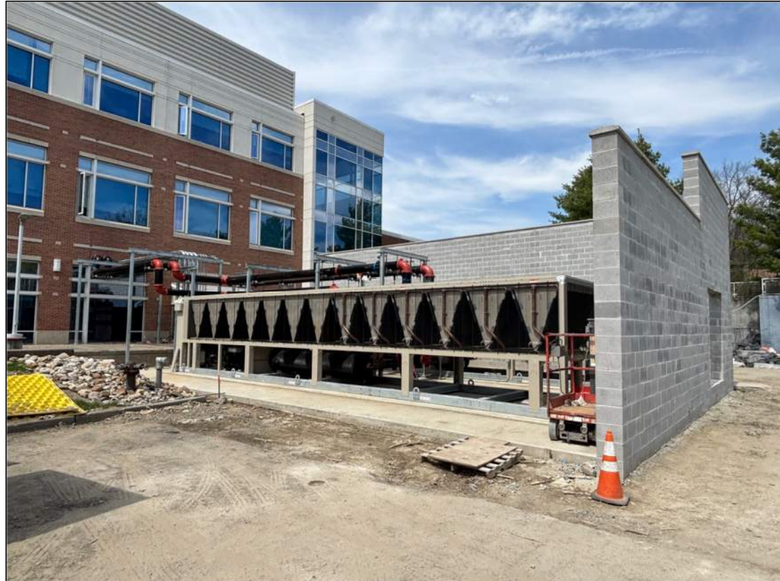
New Outdoor Chiller – 4/16/26
