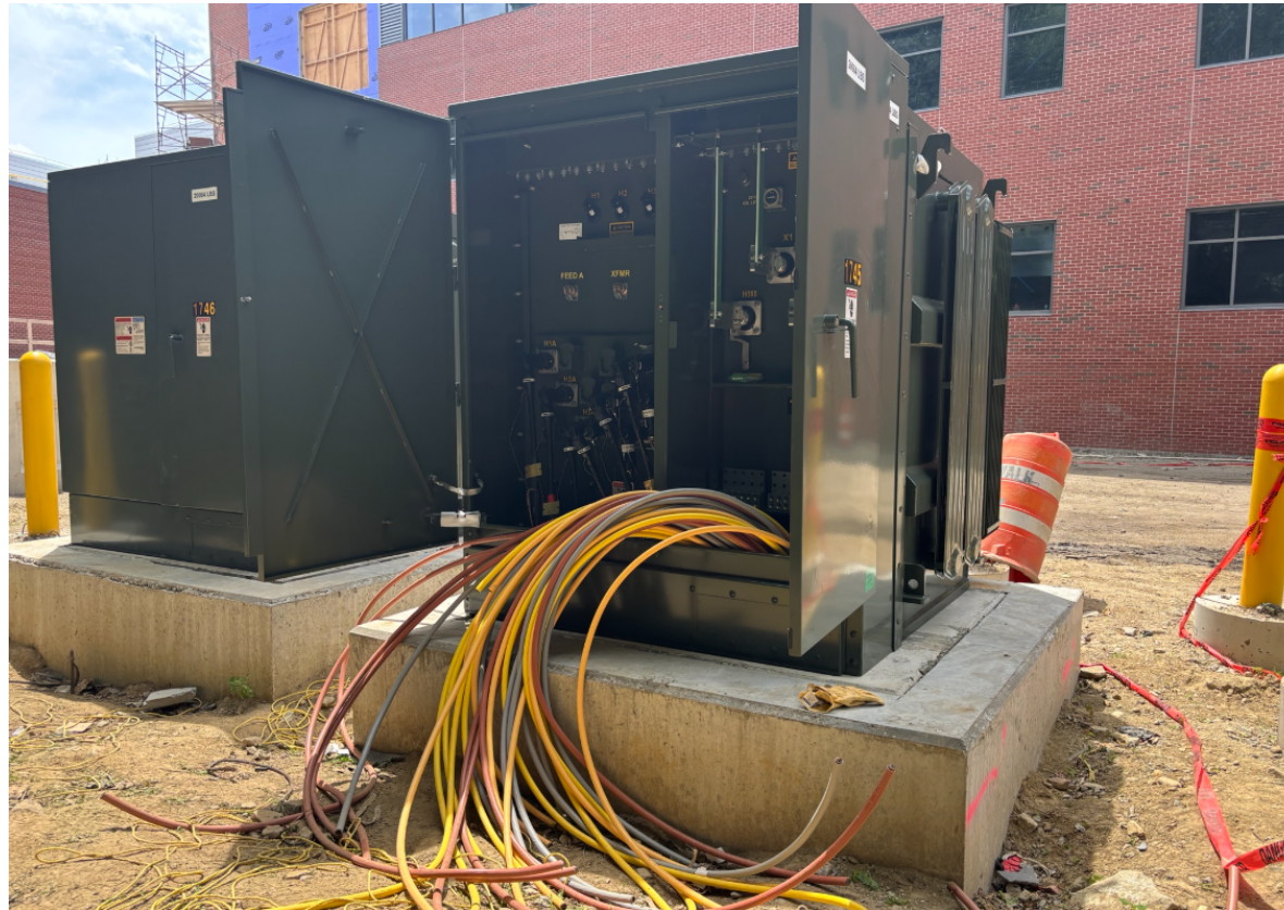
New Electrical Service – Transformers and Primary Cabling – 6/19/26
