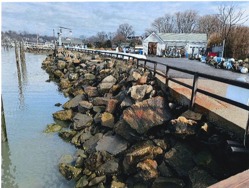
Southern Section of Seawall Facing North From Southern Deck, Photo Taken March 6, 2025
