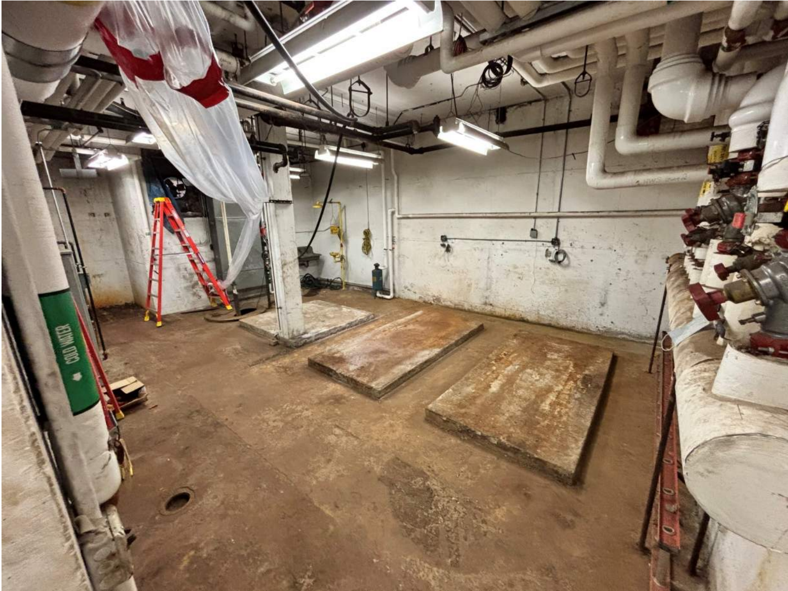
Rowayton – Boiler Room – 7/23
