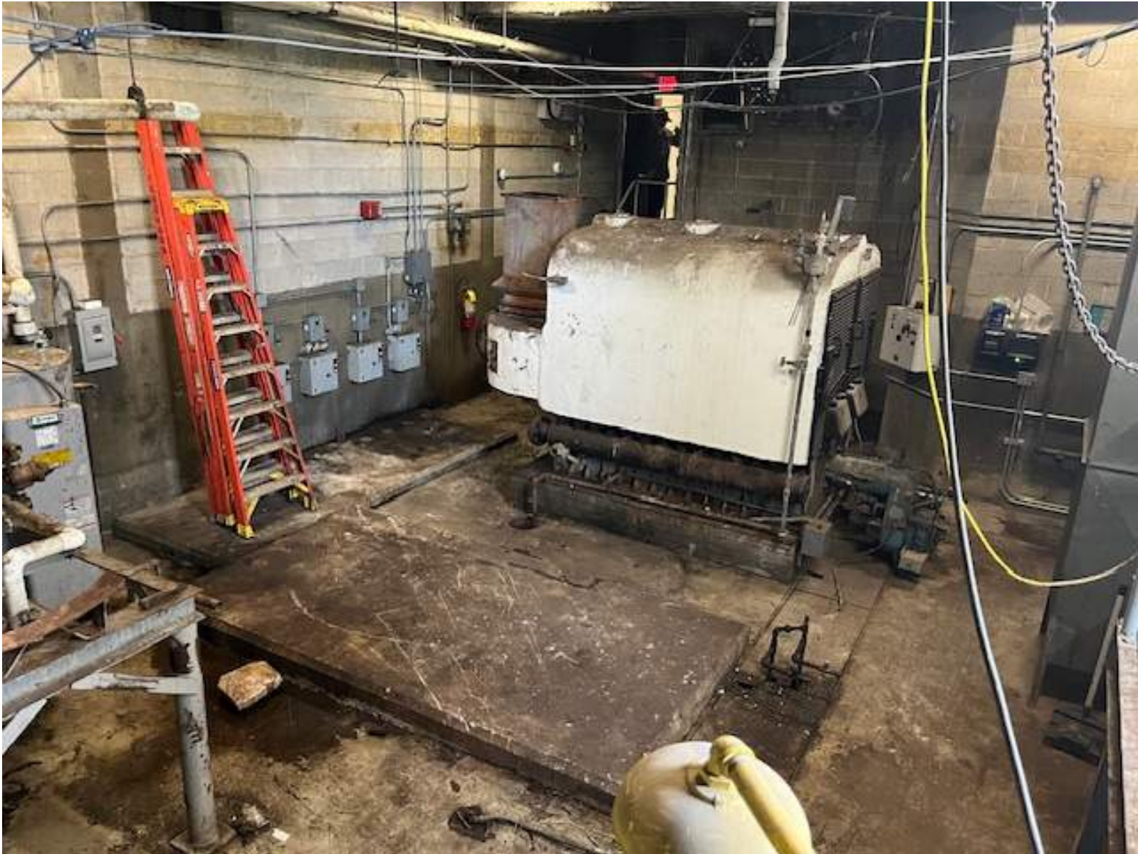
Silvermine – Boiler Room – 7/29
