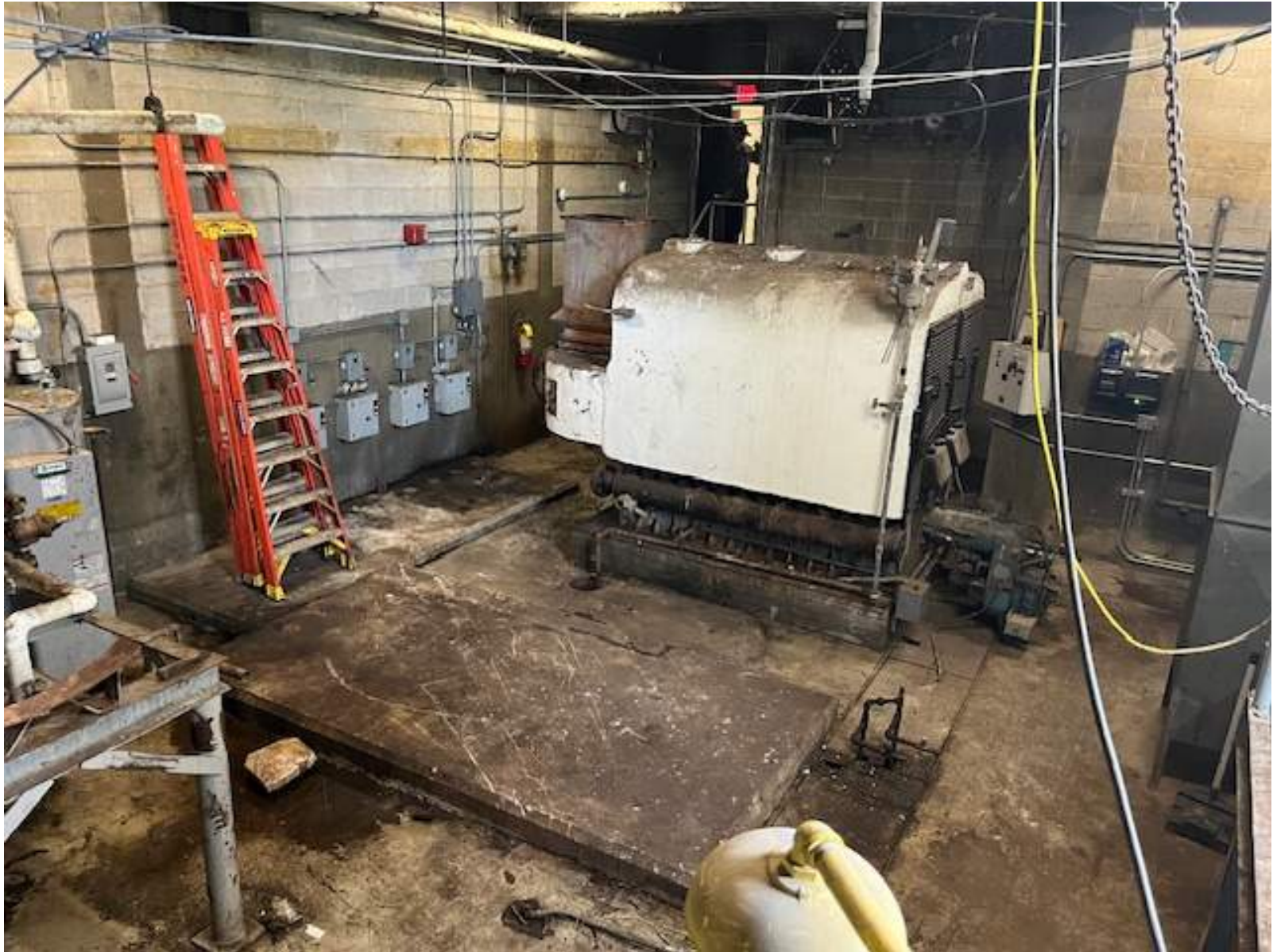
Silvermine – Boiler Room – 7/29
