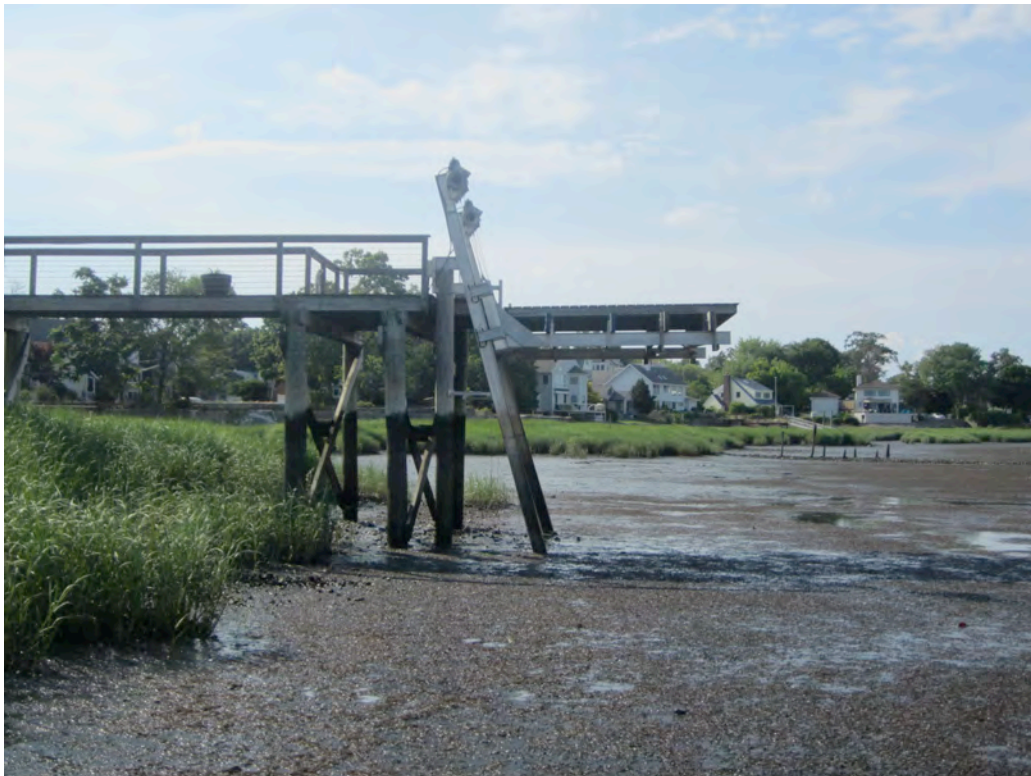
2. VIEW LOOKING NORTH TOWARDS PIERHEAD AND BOAT LIFT. NOTE UNAUTHORIZED PLATFORM ATOP BOAT LIFT, LIMIT OF TIDAL WETLAND VEGETATION, AND TYPE OF SUBSTRATE BELOW.
