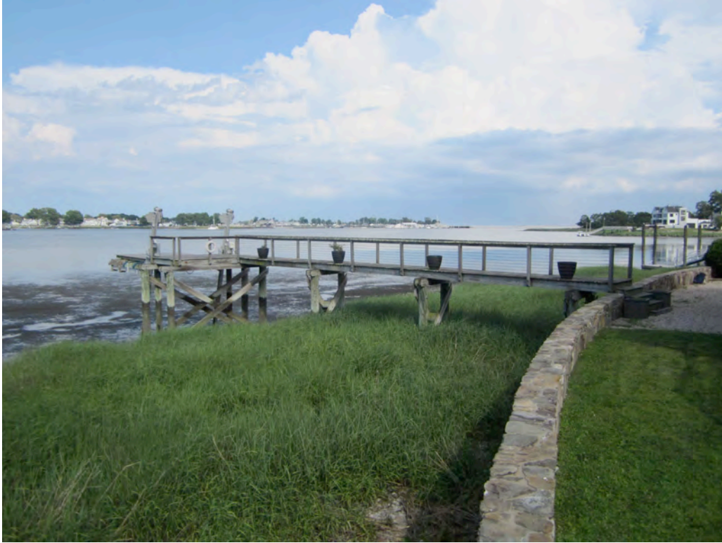
1. VIEW FROM ATOP SEAWALL LOOKING SOUTHEAST TOWARDS PIER TO BE MODIFIED. NOTE EXTENT OF INTERTIDAL WETLAND VEGETATION.
