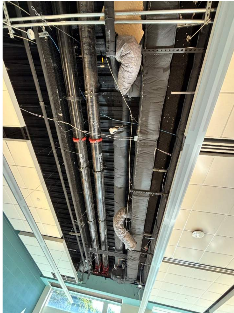
Brien McMahon High School – New Chiller Piping Entering Cafeteria – 8/20/25
