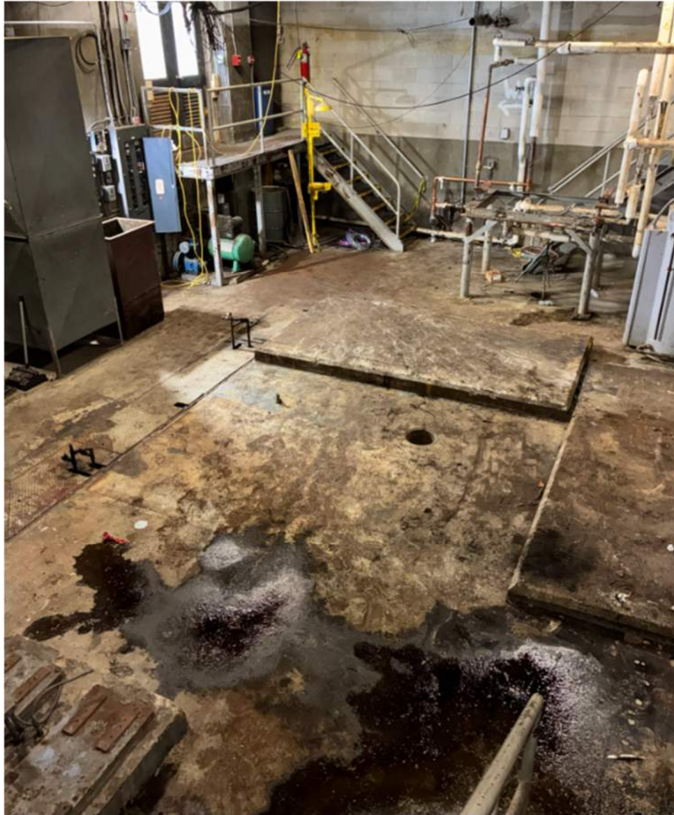
Silvermine – Boiler Room – 8/20/25
