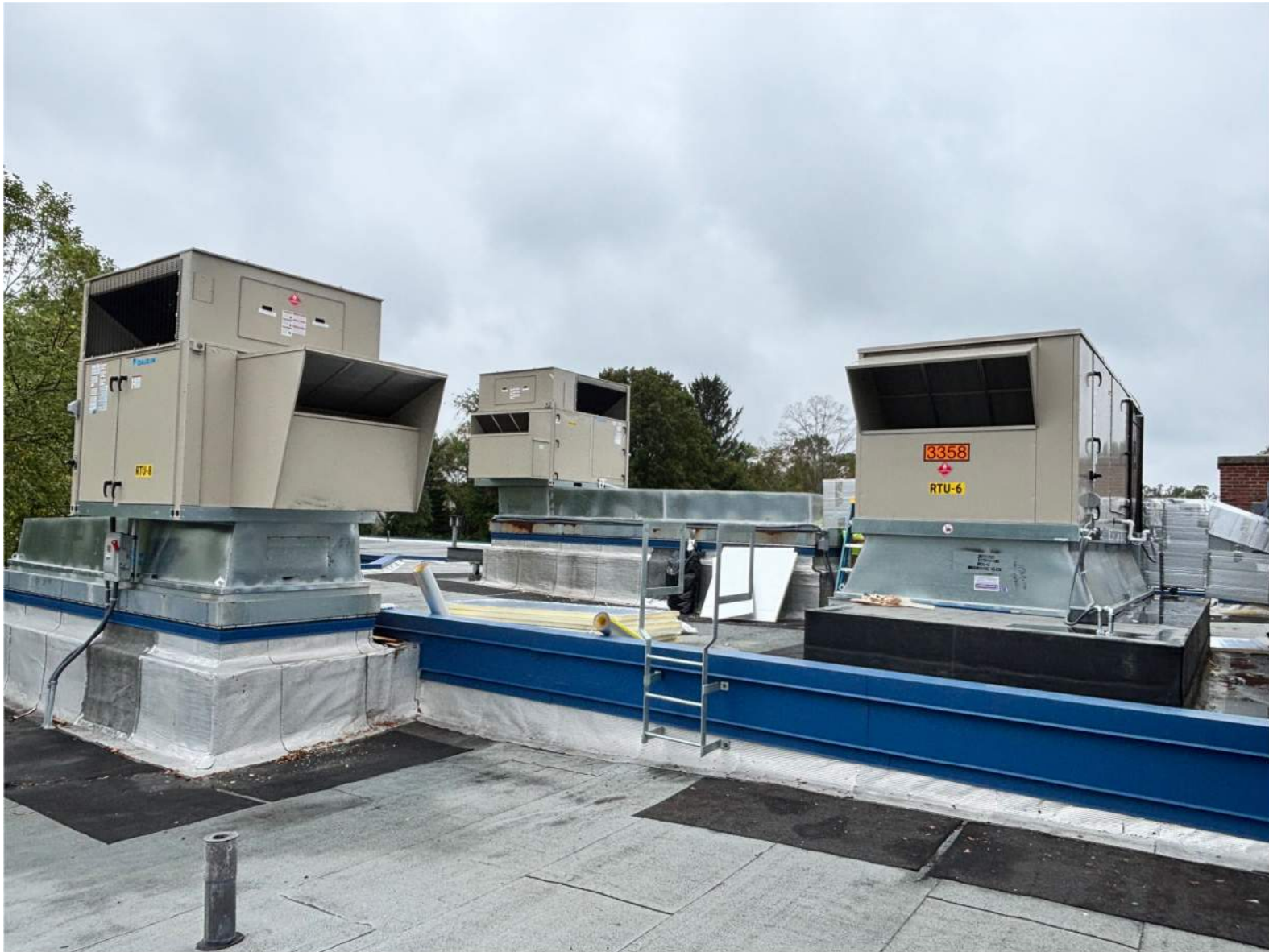
Brookside – Roof Top Units – 09/24/25
