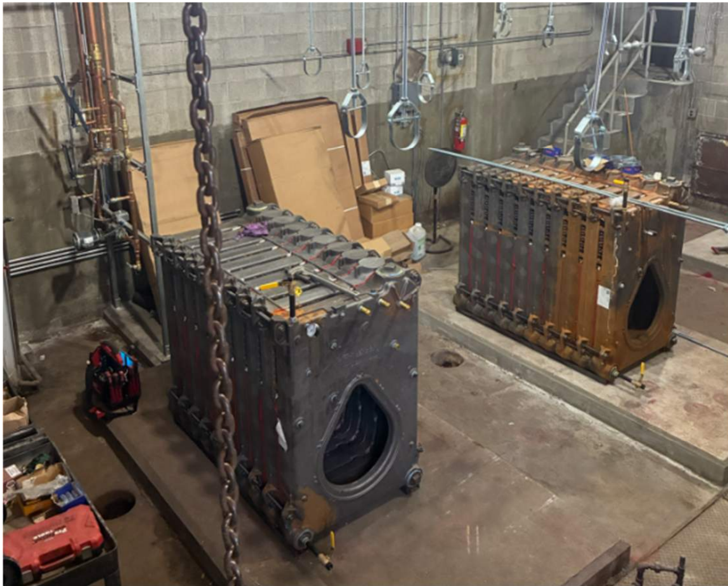
Silvermine – Boiler Room – 9/24/25
