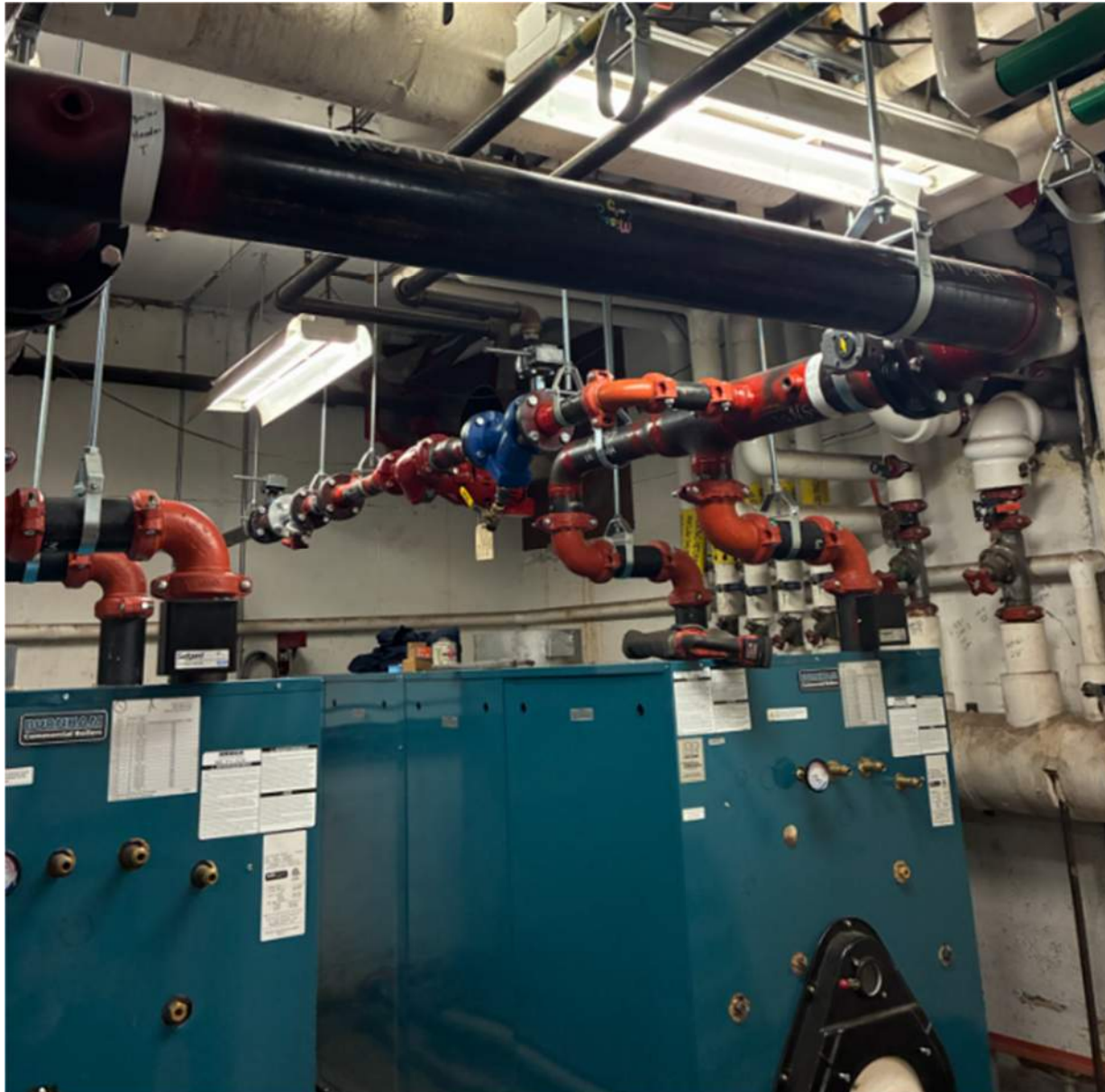
Rowayton – Boiler Room – 9/19/25
