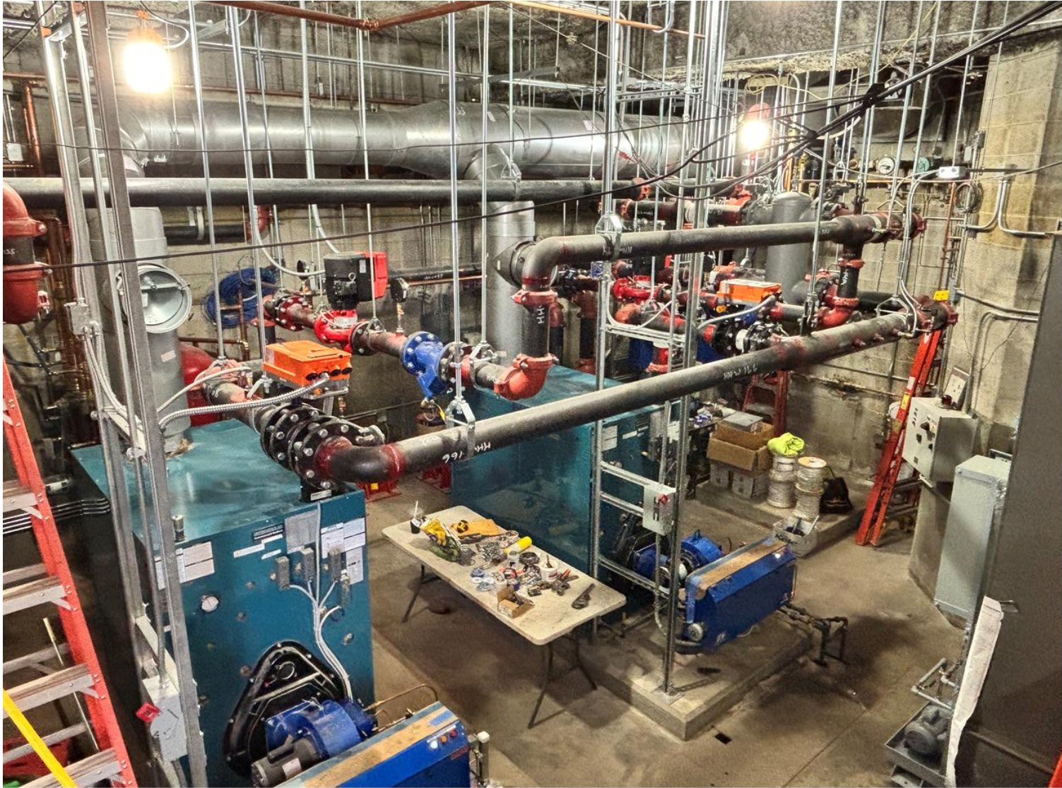
Silvermine – Boiler Room – 10/16/25
