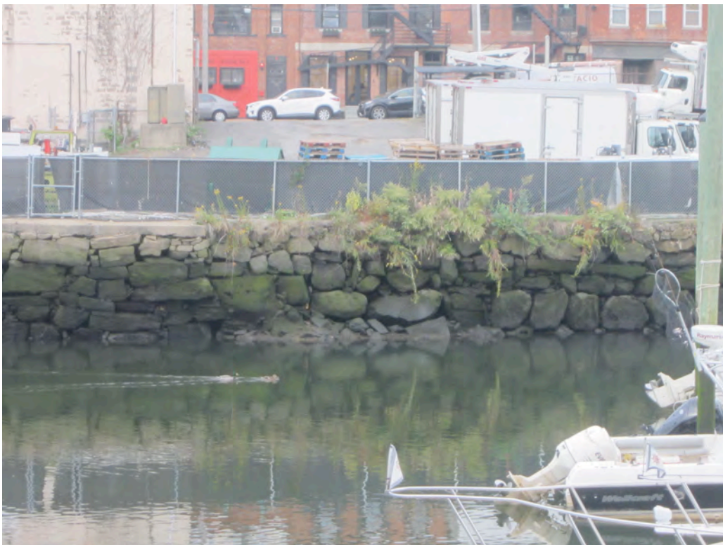
4. VIEW FROM OPPOSITE SHORE LOOKING WEST TOWARDS AREA OF SEAWALL DETERIORATION. NOTE VOIDS IN FACE OF SEAWALL AND AREA OF LATERAL DISPLACEMENT TO THE LEFT OF PHOTOGRAPH.
