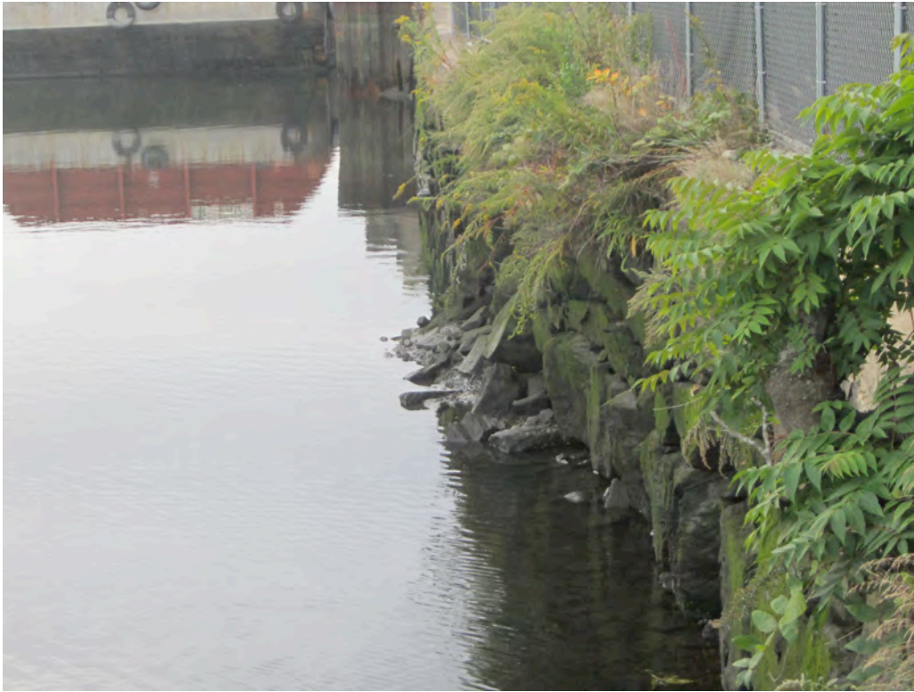
3. VIEW FROM UPSTREAM ADJACENT PROPERTY LOOKING SOUTH TOWARDS AREA OF DETERIORATION. NOTE LOOSE STONES AT BASE OF SEAWALL.
