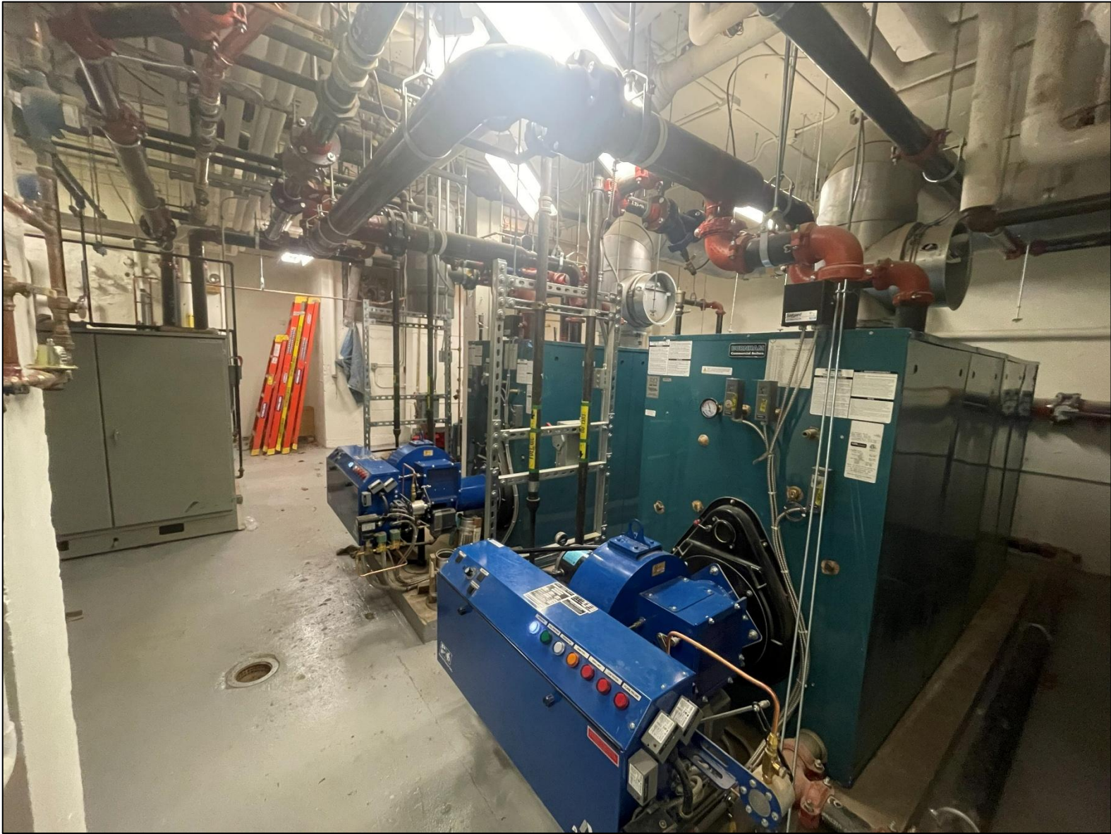
Rowayton – Boiler Room – 11/26/25
