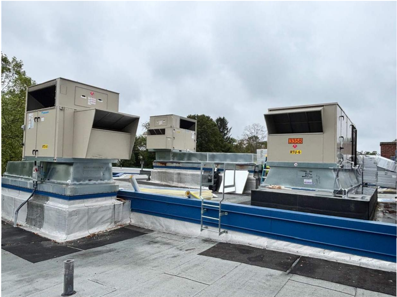
Brookside – Roof Top Units – 09/24/25
