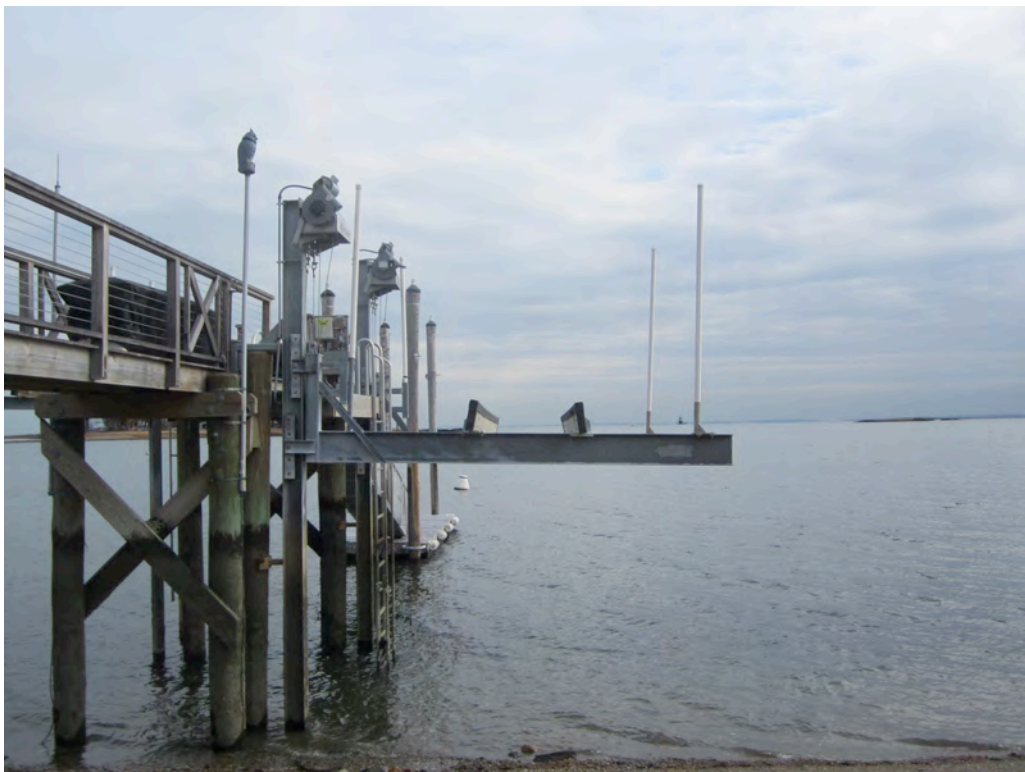
2. VIEW FROM FOOT OF REVETMENT LOOKING SOUTH TOWARDS BOAT ELEVATOR TO BE REPLACED. NOTE SLIGHT DEFLECTION OF LIFTING ARMS.
