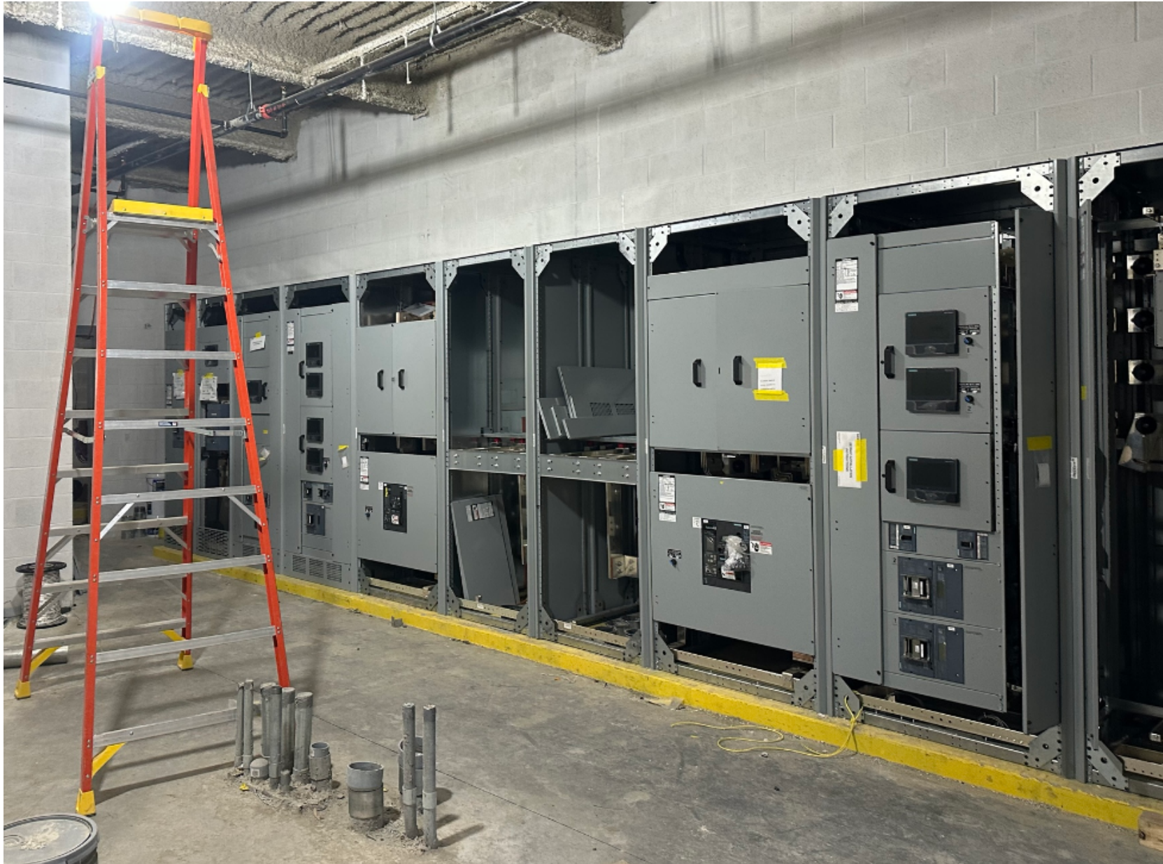
Electrical Room Equipment 1/23/25
