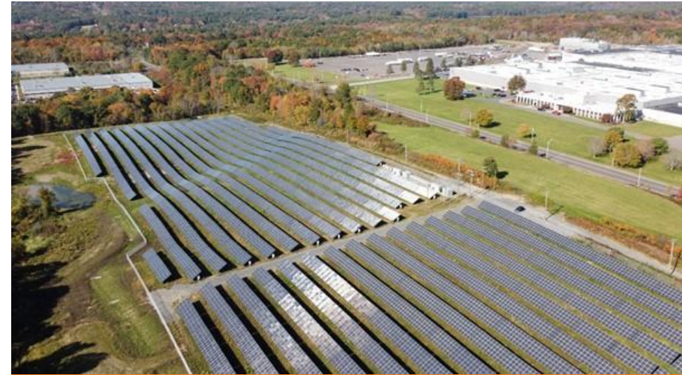
Bristol Solar One: 4,124 kW DC
