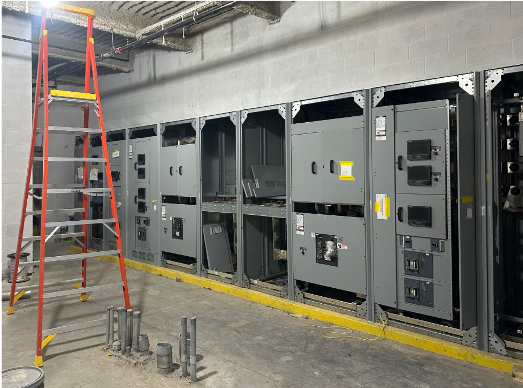
Electrical Room Equipment 1/23/25
