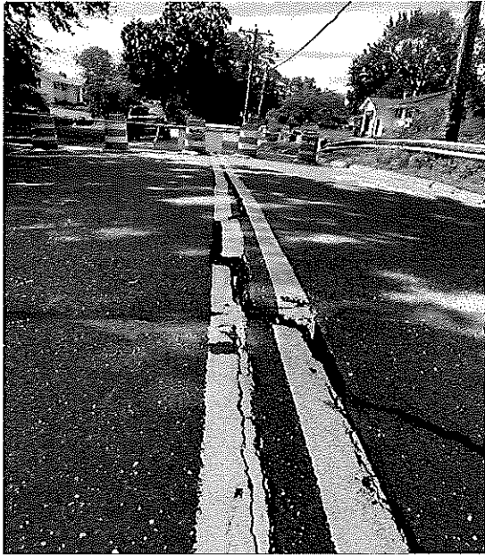
Photo # 1: Formation of 10'-15' x 2"± wide crack on pavement along center of road above the limits of the bridge.
