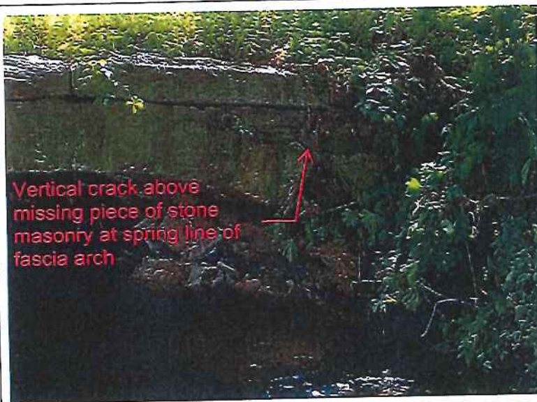
Photo # 5: Collapsed section of the stone arch located at the northwest corner of the bridge. Note that the fascia arch is hanging mid-air unsupported, which has resulted in a vertical crack above where a stone masonry is missing.
