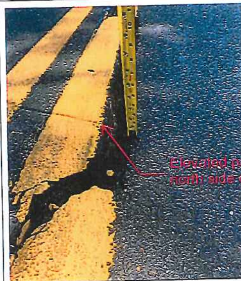
Photo # 2: Approx. up to ½" elevation differential between the north and south sides of the pavement crack.
