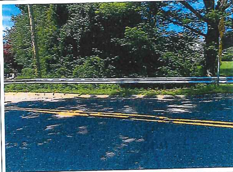
Photo # 4: View from the south side of road of noticeable "sag" in the north pavement. Also note the noticeable surface differential along the north side of the pavement crack.
