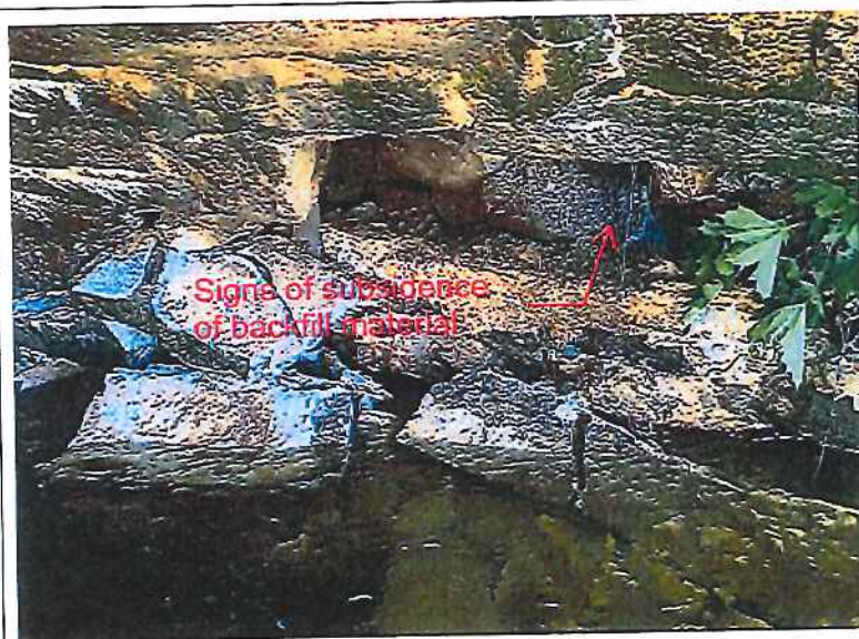
Photo # 7: Northwest collapsed section of stone masonry arch. Note signs of subsidence of backfill material.
