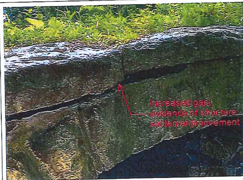
Photo # 8: A closer view of the gap between the fascia arch and the stone cap. This gap appears to have increased since the bridge was last inspected in 2018.
