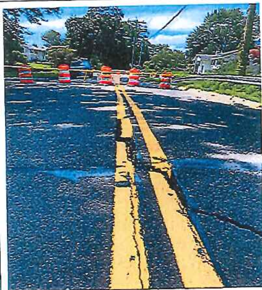
Photo # 1: Formation of 10'-15' x 2"± wide crack on pavement along center of road above the limits of the bridge.
