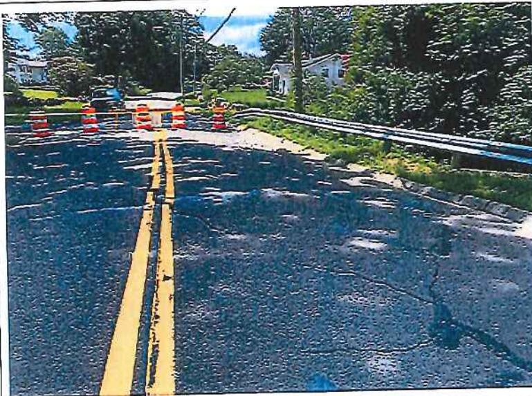
Photo # 3: Note the "sag" along the north bituminous concrete curb.
