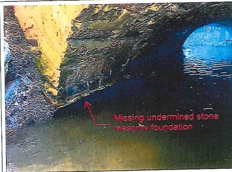
Photo # 8: Northeast section of the stone masonry arch. Note the missing masonry foundation up to approximately 10' long; stone masonry appears to have settled into the scour hole.
