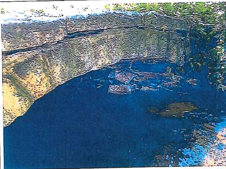
Photo # 7: North elevation view of the bridge. The fascia arch exhibits a gap approximately 2" wide between the fascia arch and the stone cap. Note the scour hole located just under inlet of the bridge.
