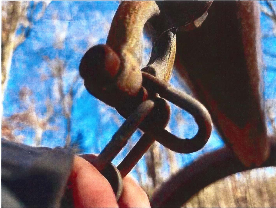
Priority 5 Safety Concern: Wear and tear showing on all chains on belt seats
